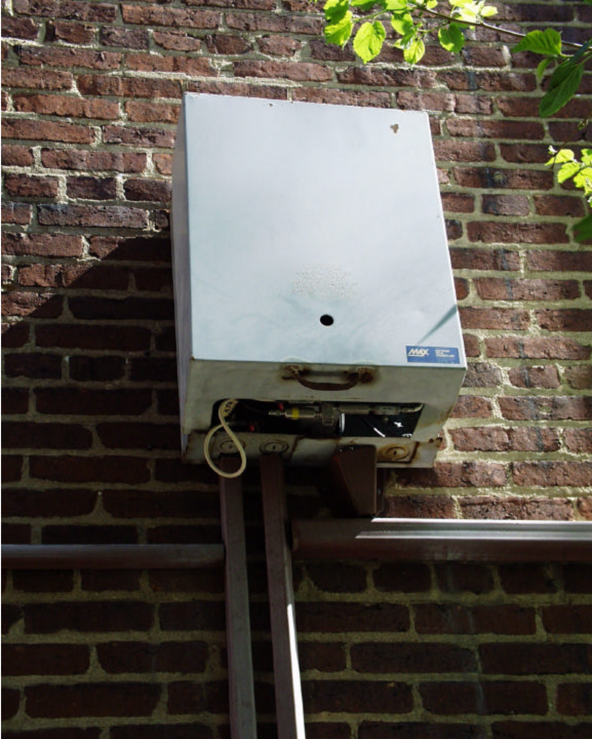
The above photograph was taken at 3620 Connecticut Avenue, N.W. on May 3, 2000. It shows an open lockbox, which contains splitters and filter traps.
