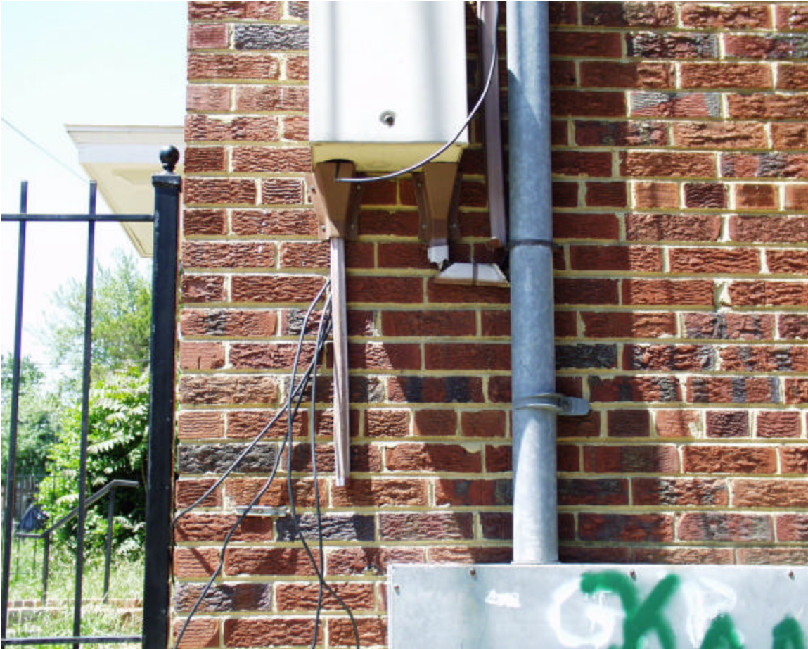
The above photograph was taken at 59 Galveston Street S.W. on May 3, 2000. It shows a lockbox with broken wiremold and loose cables.
