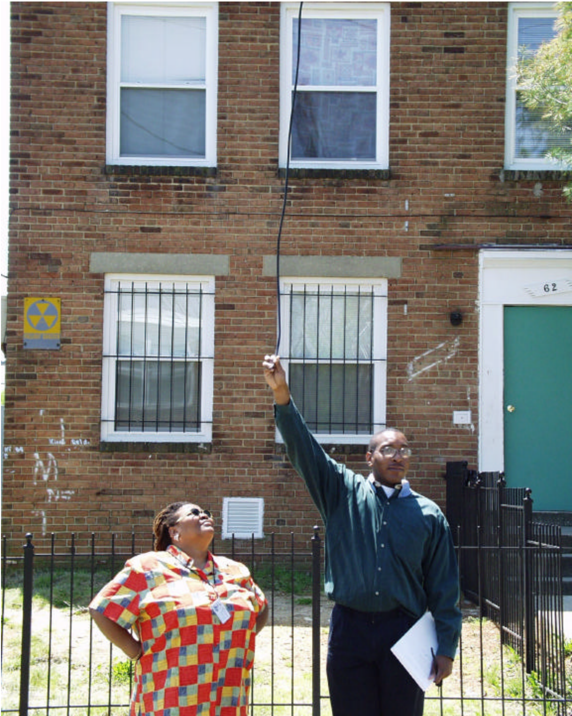
The above photograph, taken in front of 62 Galveston Street S.W. on May 3, 2000, shows a loose coaxial cable hanging low over the sidewalk area.
