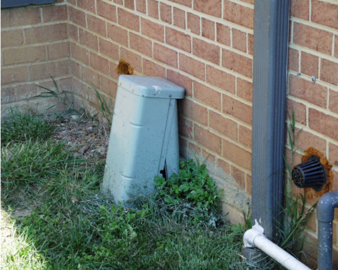
The above photograph was taken at 624 Mississippi Avenue, S.E. on May 3, 2000. It show an open pedestal, containing splitters and filter traps.
