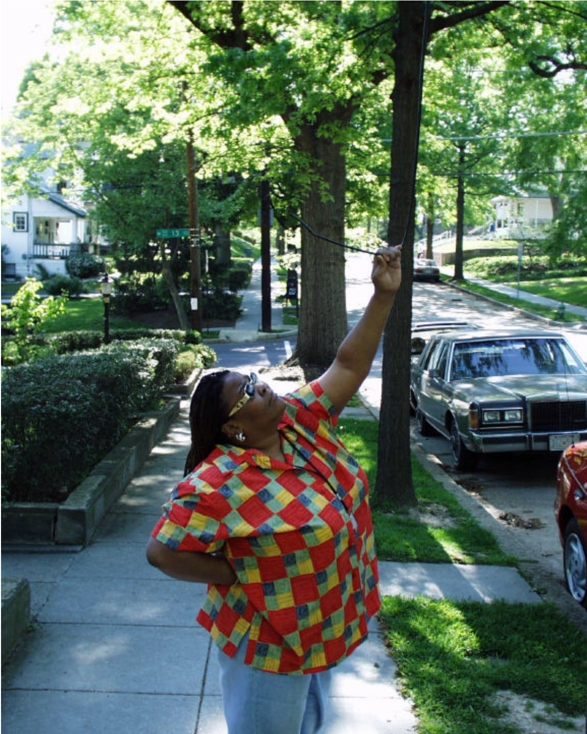
The above photograph, taken in front of 1305 Lawrence Street, N.E. on May 3, 2000, shows a loose coaxial cable hanging low over the sidewalk area.
