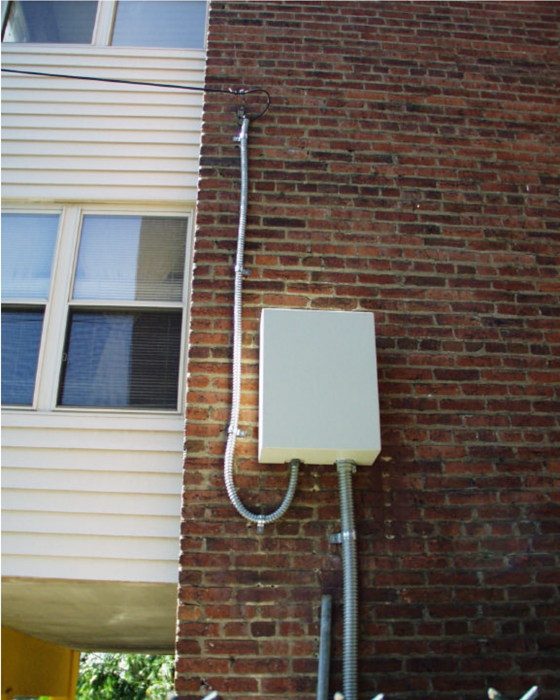
The above photograph was taken at 3618 Connecticut Avenue, N.W. on May 3, 2000. It shows a newly installed lockbox containing splitters and filter traps.
