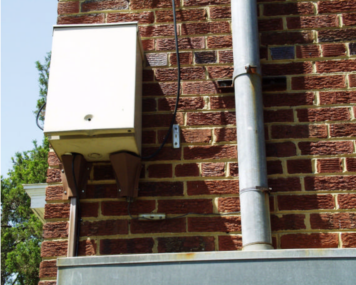
The above photograph was taken at 101 Galveston Street S.W. on May 3, 2000. It shows an open lockbox.
